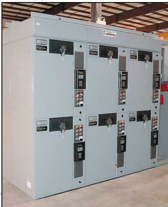
Medium Voltage Motor Control With Motor Protective Relays Per Customer Requirements
