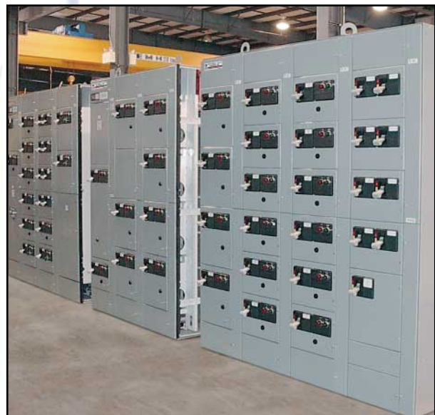
Low Voltage Motor Control Centers In Unlimited Arrangements and Flexibility
