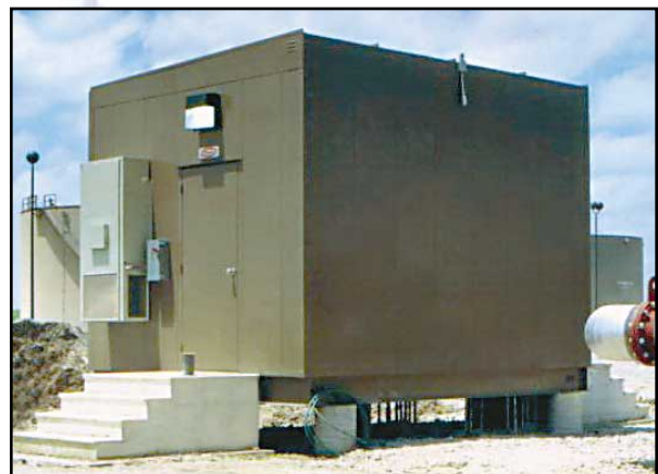
Single Wide Control Center With Motor Control Equipment
