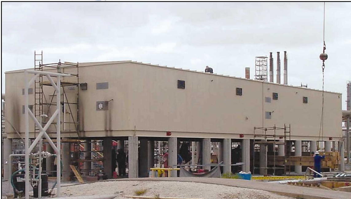
Fully Integrated Power Distribution Center Four Way Split - 32 Feet Wide By 94 Feet Long
