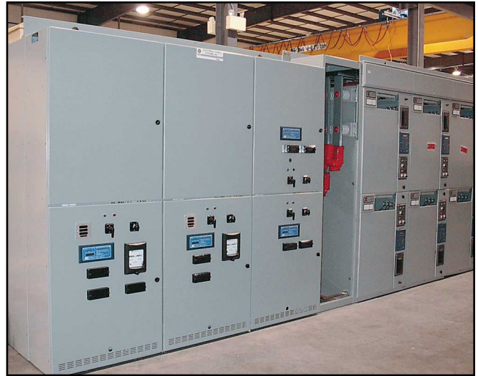
Medium Voltage Switchgear with Protective Relaying Close Coupled to Medium Voltage Motor Control with Motor Protective Relays
